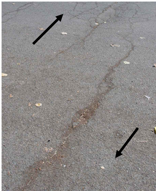
En echelon fault pattern seen in the asphalt
